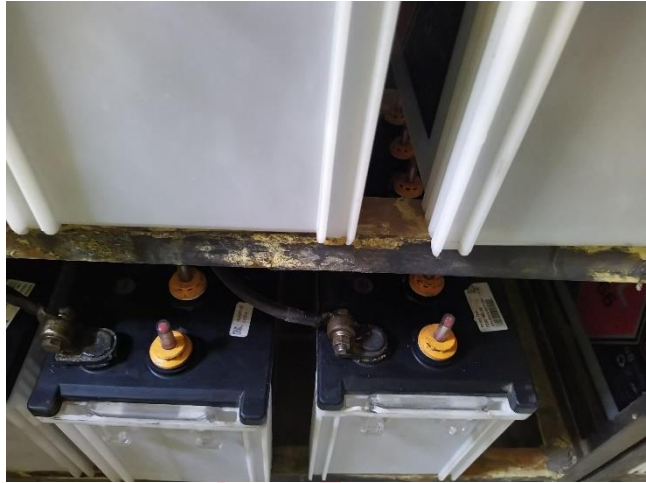
Figure 16 - Placement of battery is in danger
