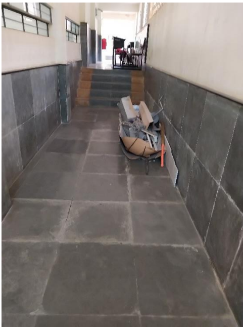
Figure 9 - absence of waste collection bins in the corridor
