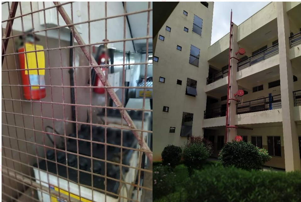
Figure 22 - No ready access to fire extinguisher.
