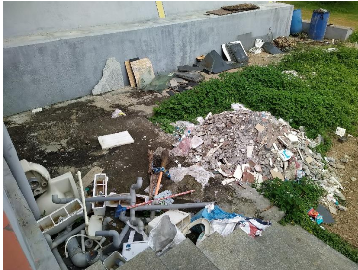
Figure 35 - Construction waste to be marked for further action
