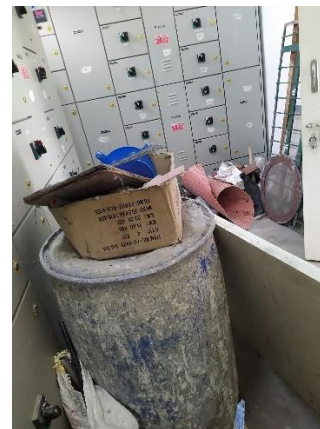
Figure 34 - Keeping waste away from Electrical room
